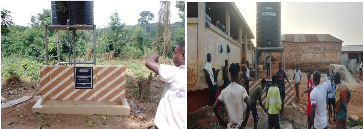
Figure 4: Completion a mechanized Bole hole with poly tank and electricity connection at Gomoa Ayanful
